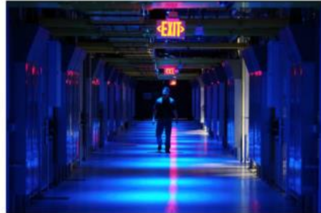
A data center in San Jose, Calif. A.I. is having a profound impact on energy demand around the world. Jim Wilson/The New York Times
